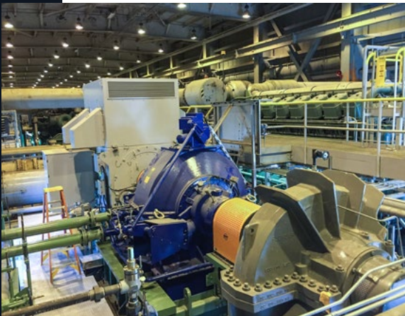
A pump, fluid coupling and motor.
